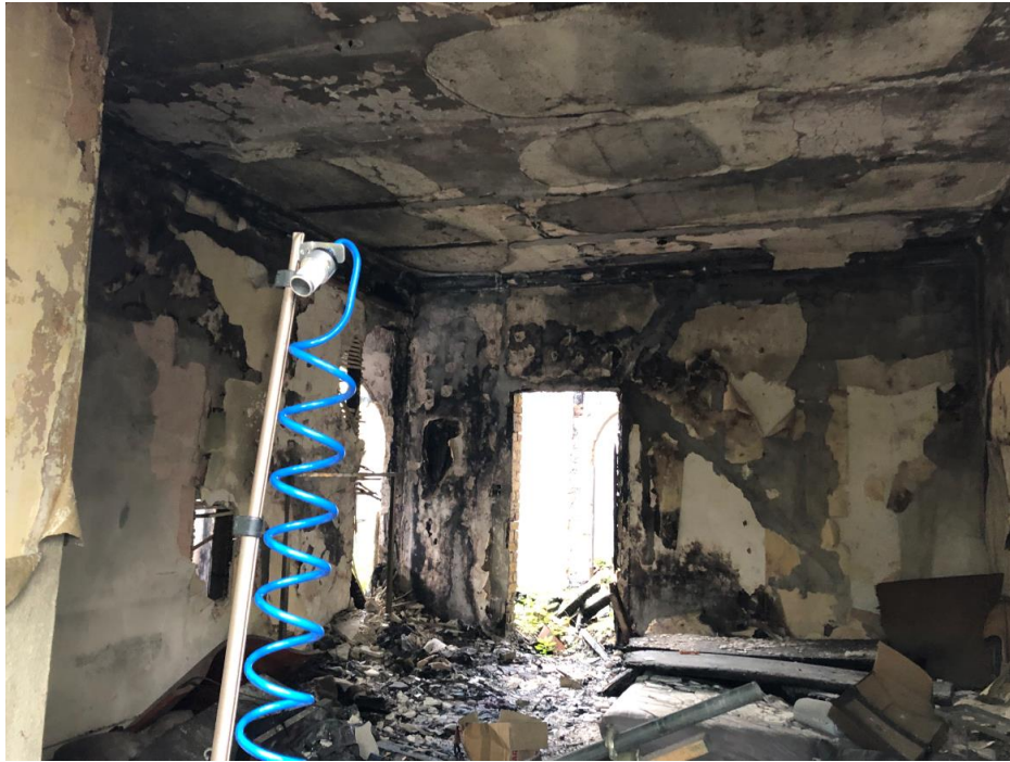
Photo 26 - Fire damage wall and water penetration through roof of Apartment 10
