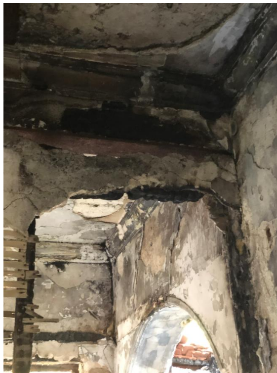
Photo 27 - Steel beam above fire damaged wall of Apartment 10
