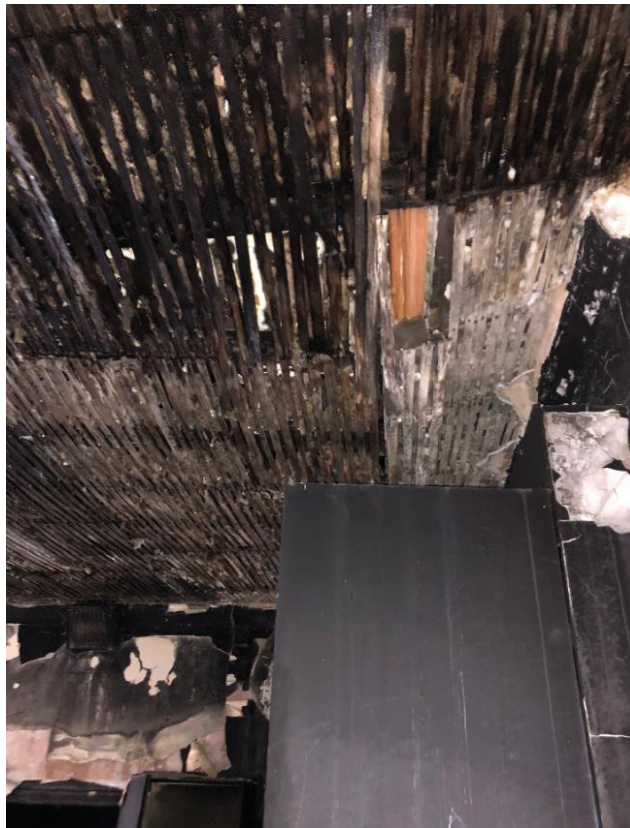
Photo 29 - sagging trimmer joist at second floor level above Apartment 9
