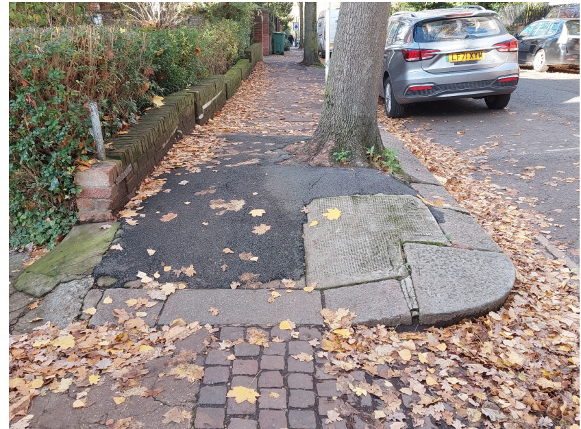
Showing where original paving materials have been removed and asphalt patching and loss of grass verges has occurred.
