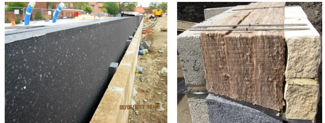
Figure 11.15 - Good examples of insulation installed on site, showing methods to eliminate gaps (wedging and overfilling). Left: Goldsmith street © Etude, Right: © Green building store.
